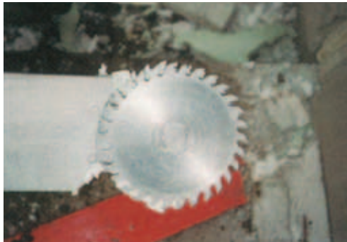
Fig. 18 – Repair work at a two-layer aerated concrete masonry wall with a double-sided saw blade on a 5 metre long blade [7.14]
