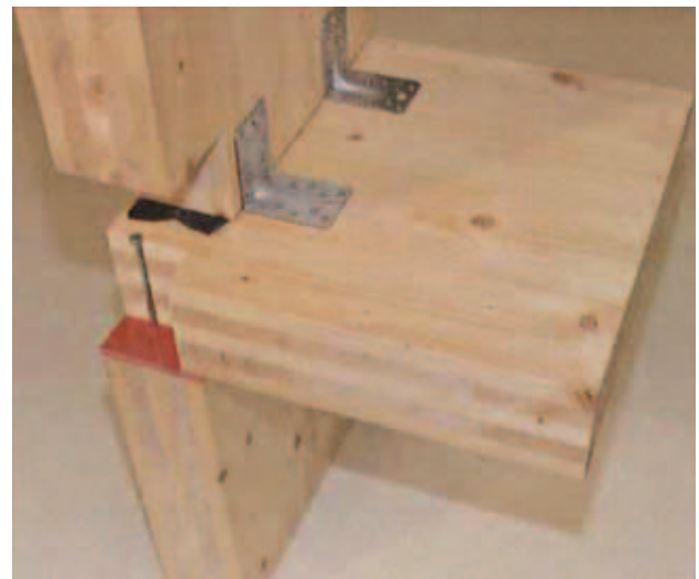
Fig. 17 – Bearing by Getzner (red, bottom) and Trelleborg (black, top) as possible improvement of the flank [7.7]
